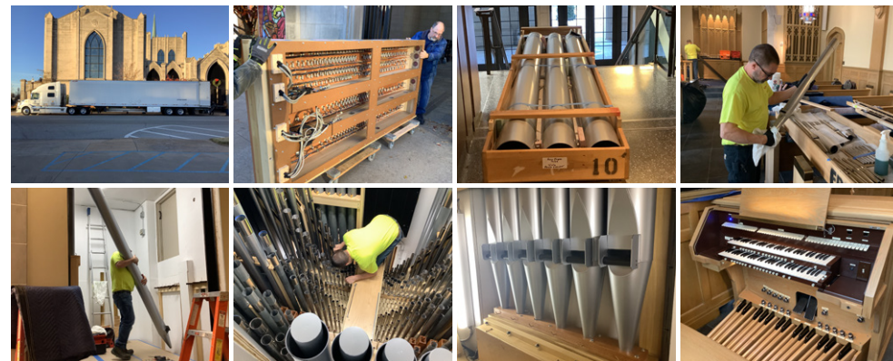
The Kerr Chapel organ installation involved significant construction, mechanical and electrical work, precision carpentry and acoustic expertise.
